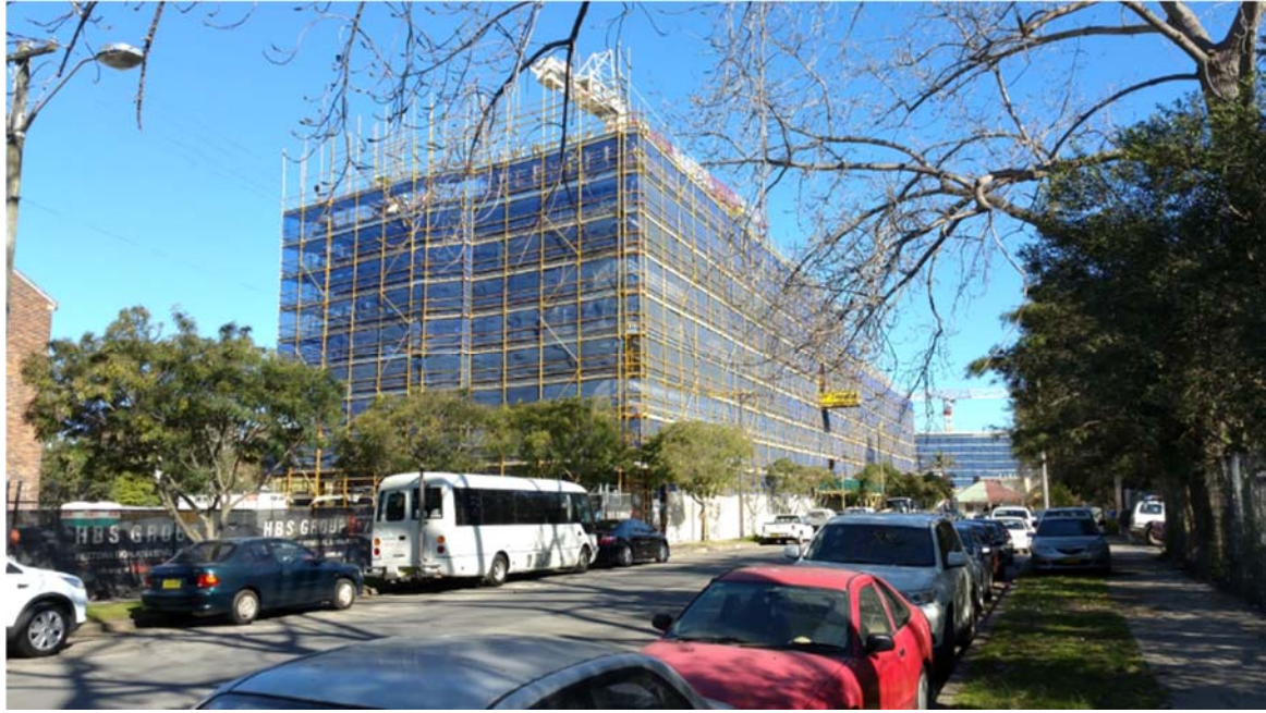
Figure 6: CityWest Housing affordable housing buildings under construction to the south-east of the site.
